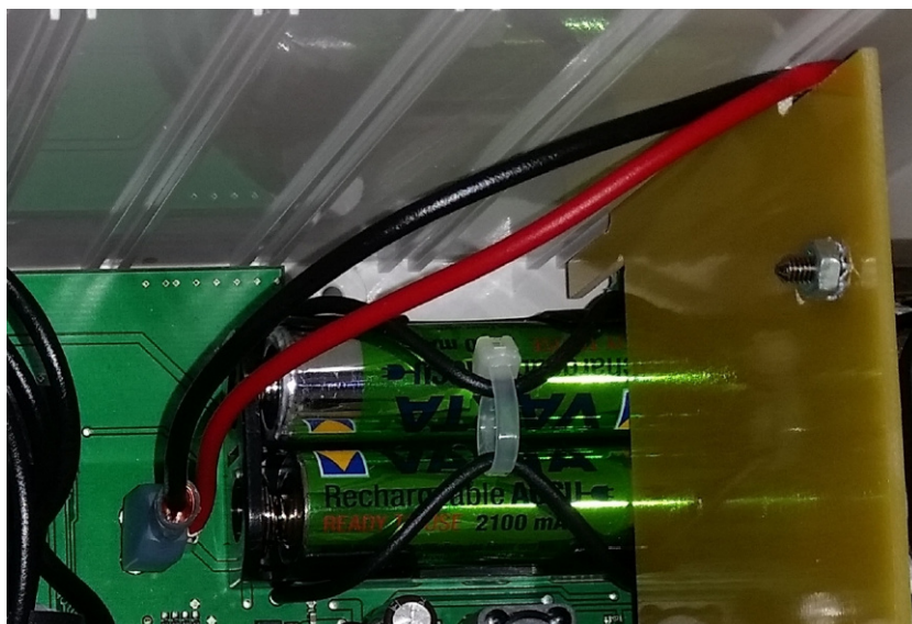
Fig. 2: +24VDC red cable and Ground black cable
